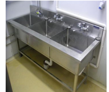
Three Compartment Dish Washing Sink
