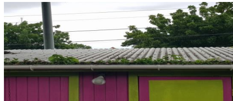
- Roof gutter holding leaves and debris
